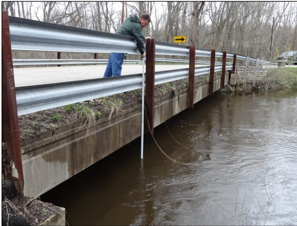
Figure 60. Example of how water surface elevations were measured with reference to the low chords of the bridges during the April, 2013 flood. This is at Sink Rd. (photo provided by Robert Frank).
