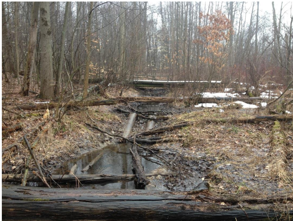
Figure 50. The old crossing above the pond - note the two old pipes in the bed
